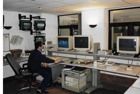
Broomy Hill WTW Control Room (2000)
