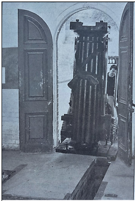
Manoeuvring the massive centre column through the narrow doors of Bay Five
