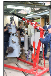
Nov 2021 Engines moved to display shed - it then took 15 months to install the engines in working order
